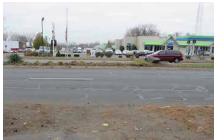
A sidewalk in poor condition along the northern side of West Street opposite the Pride Service Station.
