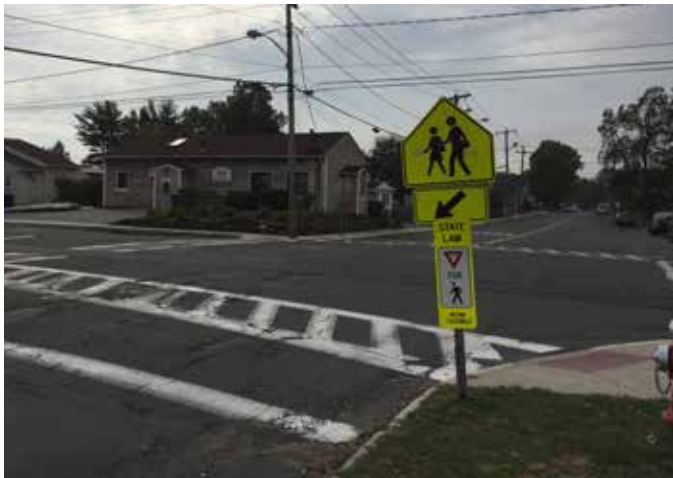
Missing stop sign at the intersection of Norman Street and Cold Spring Avenue.
