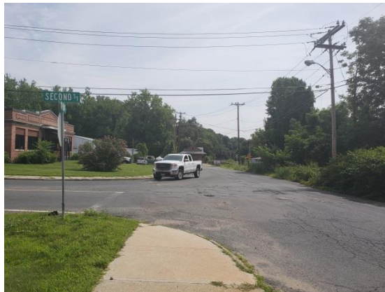
Figure 5: Pavement Condition and Curbing
