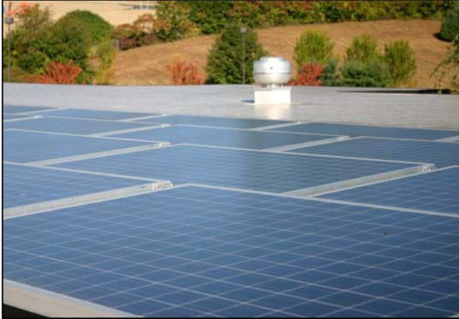
Solar Panels on the JFK Middle School in Northampton
