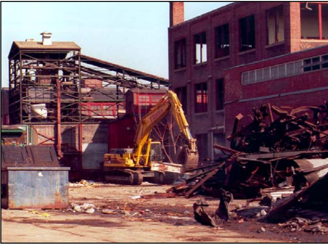
Demolition of the HB Smith Boiler Company, Westfield. Photo provided by Tighe & Bond
