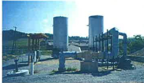
Two enclosed methane flares at the I-95 Landfill in Michigan
